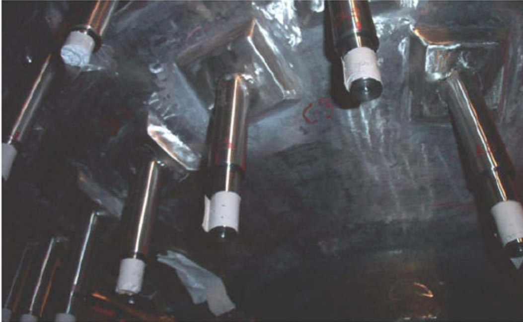
Photo 4: Pressurizer Weld Pads and New Sleeves
