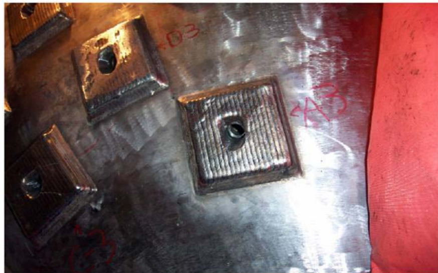
Photo 3: U2 Square Weld Pad
